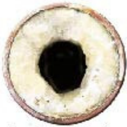
Scale buildup in a pipe, caused by hard water.
